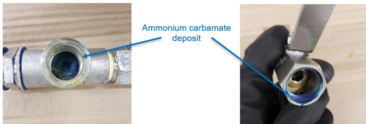
Figure 5: Ammonium carbamate deposit in unheated section of the pipeline.
